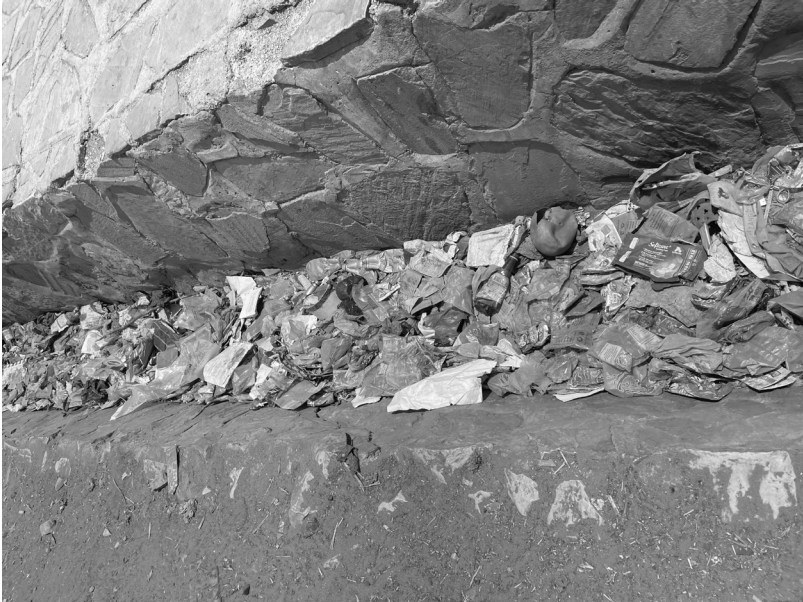
Fig. 1: Blocked sewer, Misisi, Lusaka, October 2022 (own image)
