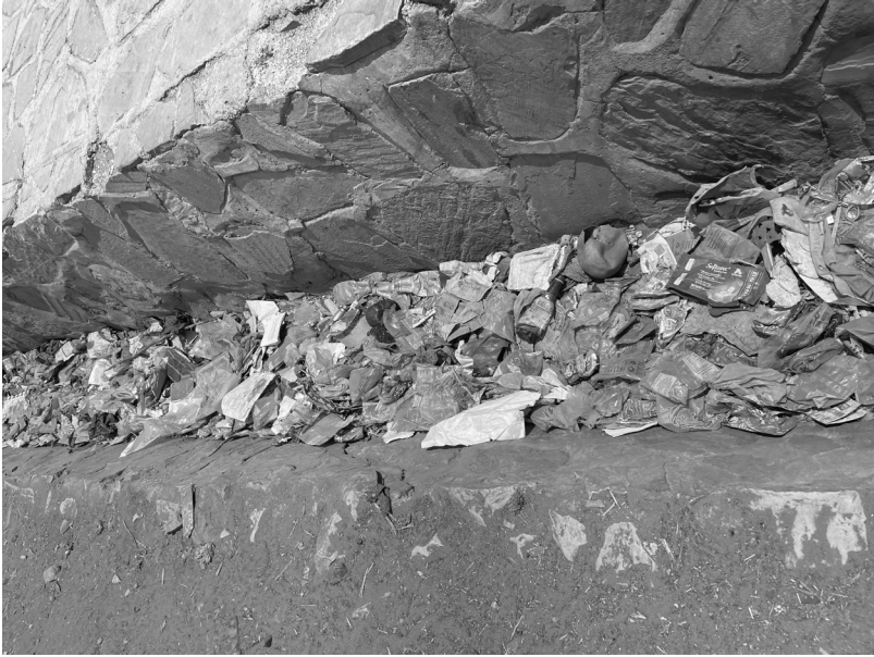
Fig. 1: Blocked sewer, Misisi, Lusaka, October 2022 (own image)
